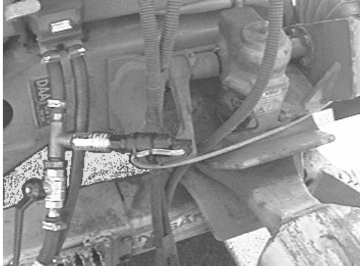
Figure 4 Control pressure transducer
