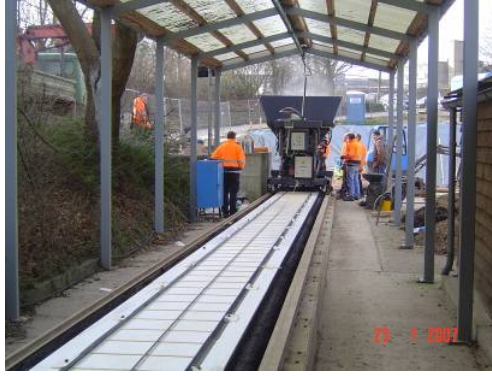
Figure 6 – Underlayer: wood plate with steel bars left and right before paving, paver in the background
