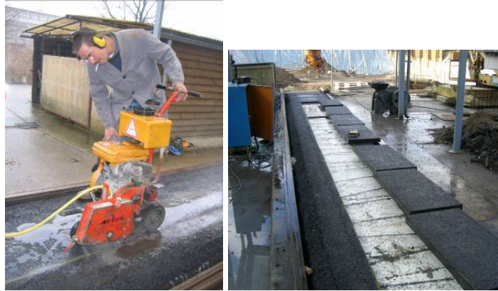
Figure 7 – After paving: cutting out slabs to be glued later into the caskets
