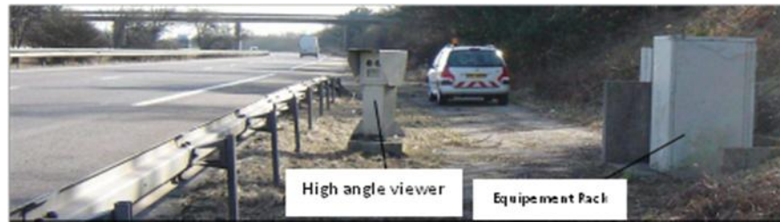
Figure 1 - Weighing equipment for heavy vehicle on the circulating road.
