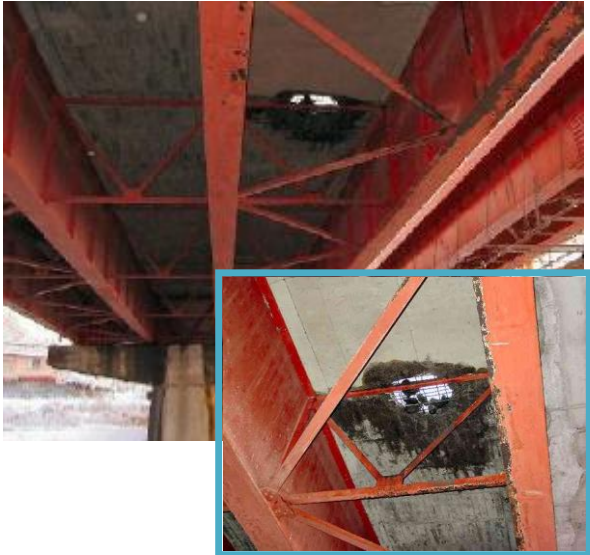
Figure 5 - Bridge Deck Requiring Treatment
